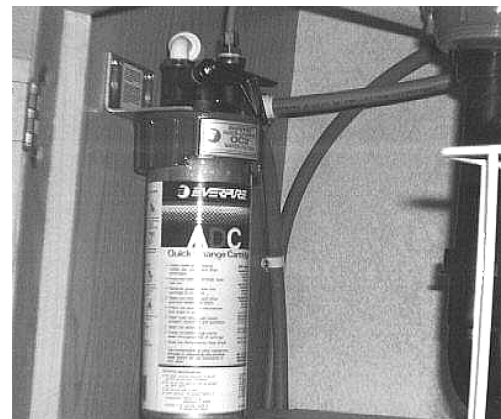
Water Filter Assembly - Below Galley Sink
