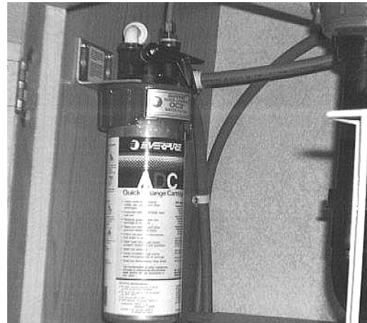
Water Filter Assembly - Below Galley Sink
