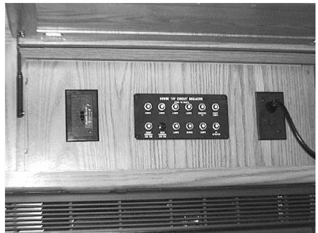
House 12-Volt Breaker Panel
