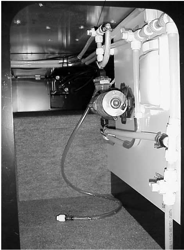
Winterizing Valve & Hose in Right Front Compartment
