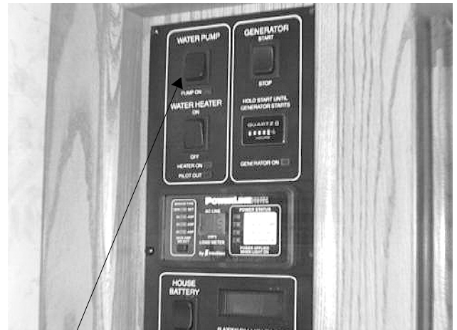
Water Pump Switch
