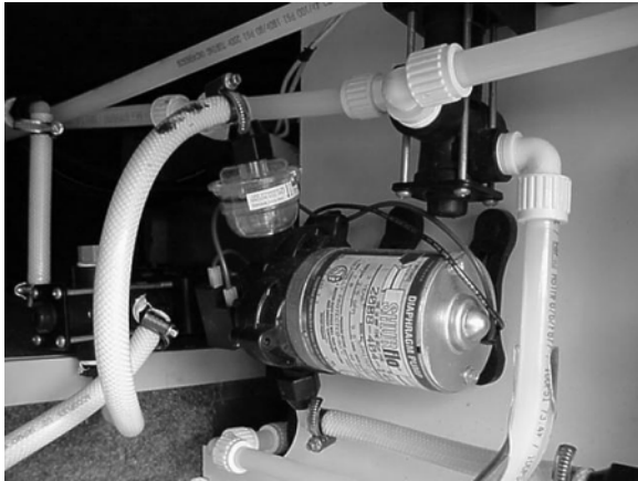
Water Pump and Filter
