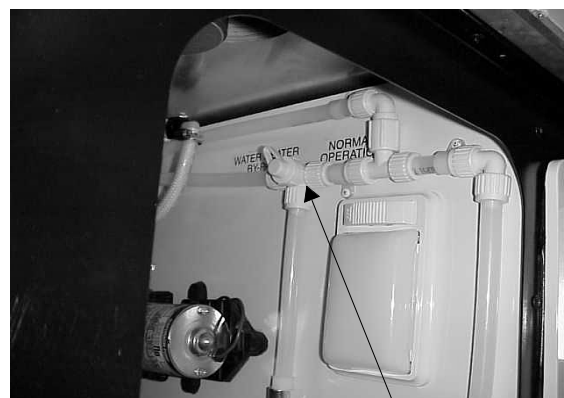
Water Heater Bypass Valve
