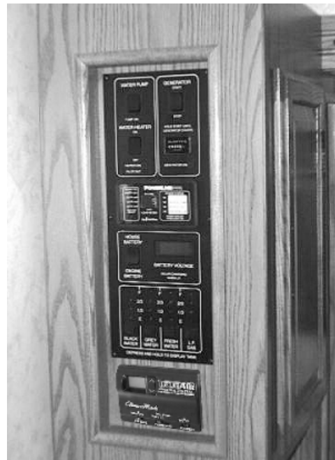
One Place Monitor Panel
