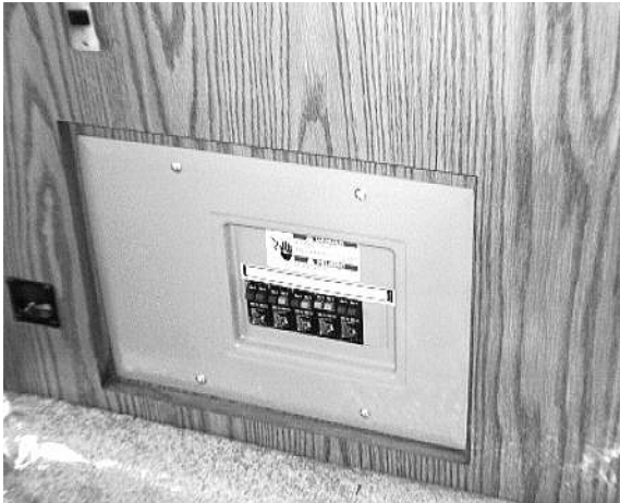
House 110-volt Breaker Panel
