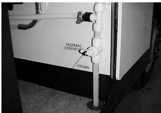
Water Line Drain Valve
