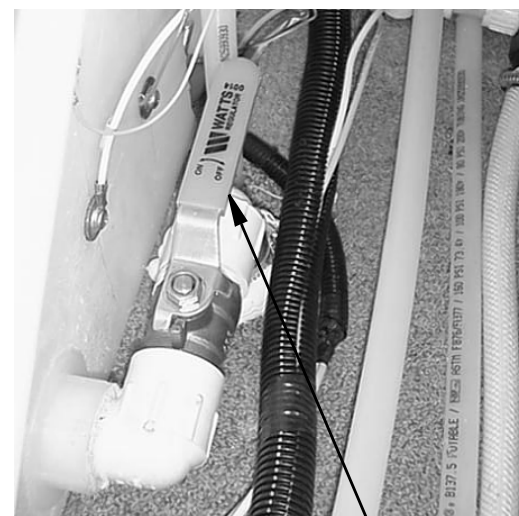
Water Tank Drain Valve (Typical)
