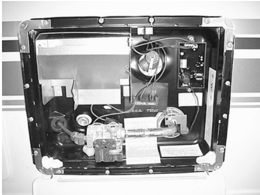
Water Heater Exterior Service Access
