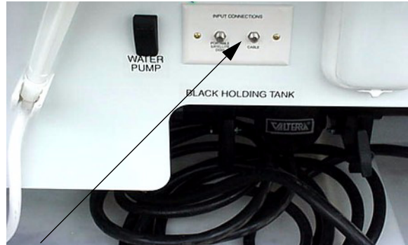
Cable TV Input Hook-Up in Utility Compartment
