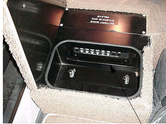
Chassis/House 12V Circuit Breakers behind cover panel in floor compartment between front seats.
