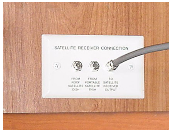
Interior Connection for Satellite Receiver (in video cabinet)
