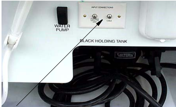
Cable TV Input Hook-Up in Utility Compartment
