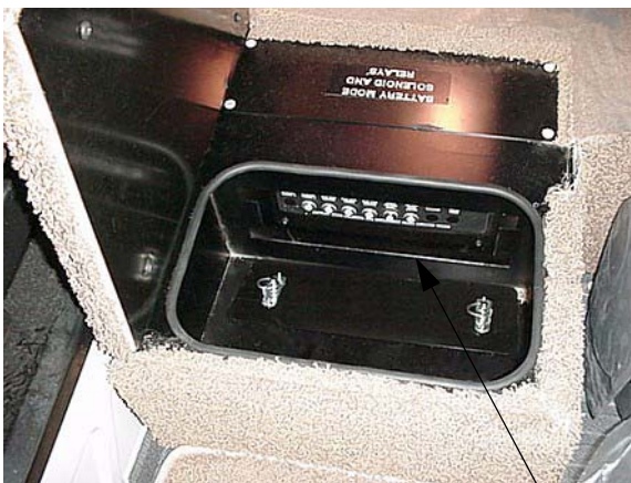
Chassis/House 12V Circuit Breakers behind cover panel in floor compartment between front seats.
