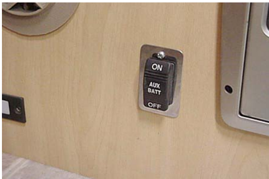
Aux. Batt. Switch - typical (Near entrance door)
