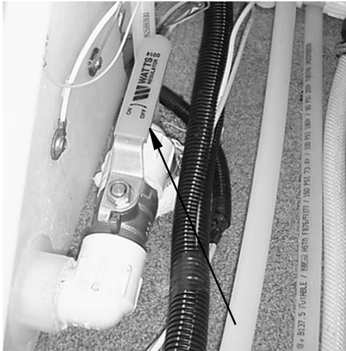
Water Tank Drain Valve (Typical)
