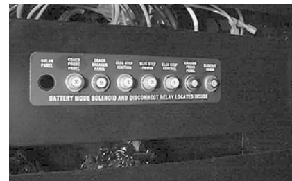
Chassis and House 12V Breakers (cover off)
