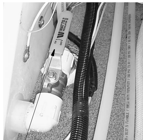
Water Tank Drain Valve
