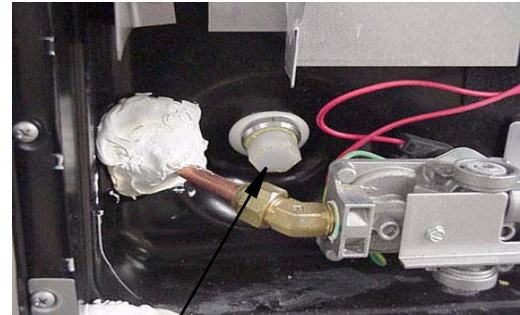
Water Heater Drain Plug Remove with socket.
