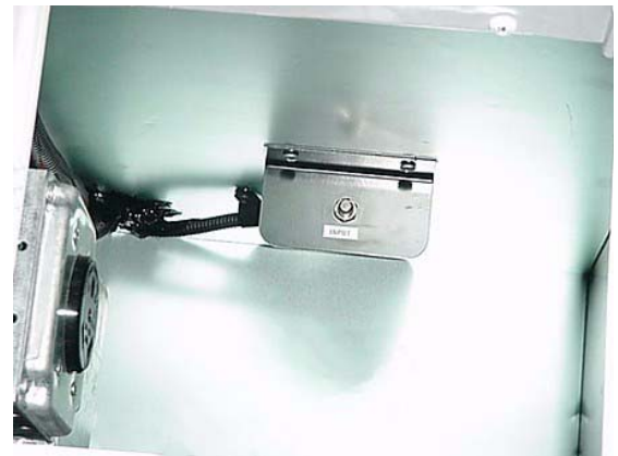
Cable TV Hook-Up in Utility Compartment
