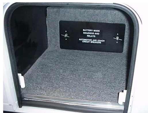
Chassis and House 12V Breakers in exterior storage compartment (remove cover to access)
