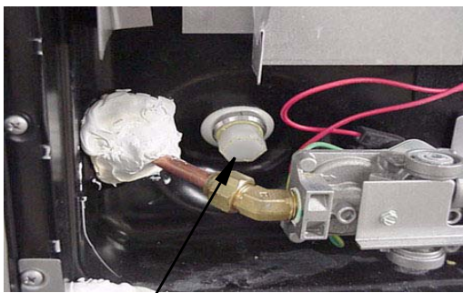
Water Heater Drain Plug Remove with socket.
