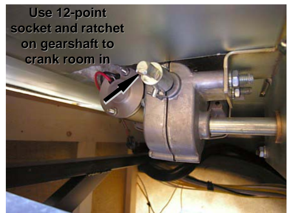
Rear Slideout Room Motor/Gear Assembly (view from access panel at foot of bed)
