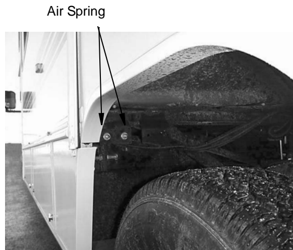
Rear Air Spring Valves (Located inside left rear wheel well)
