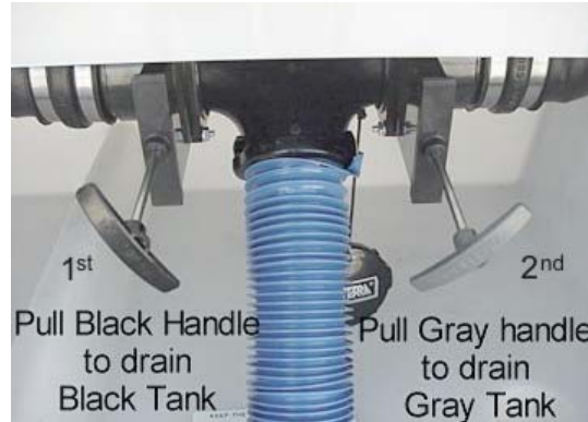
Holding Tank Dump Valves -Typical View
