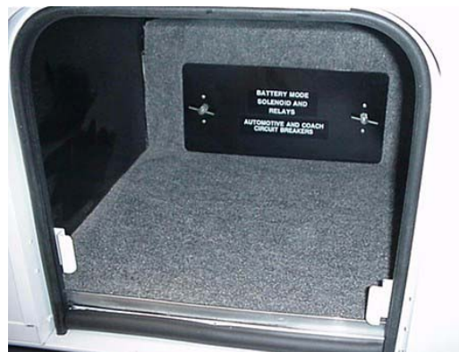
Chassis and House 12V Breakers in exterior storage compartment (remove cover to access)
