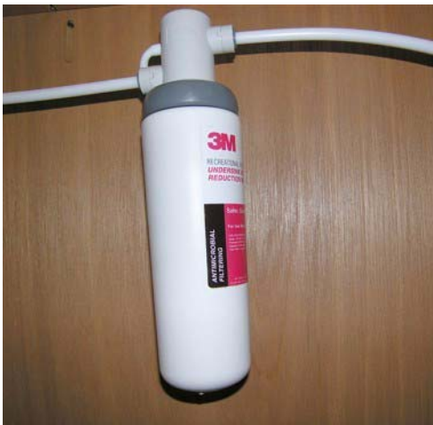
Cold Water Filter Assembly below Galley Sink (Hot waterline is not filtered)
