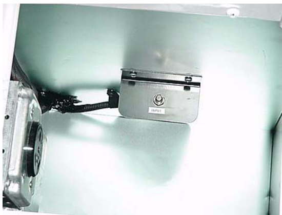
Cable TV Hook-Up in Utility Compartment
