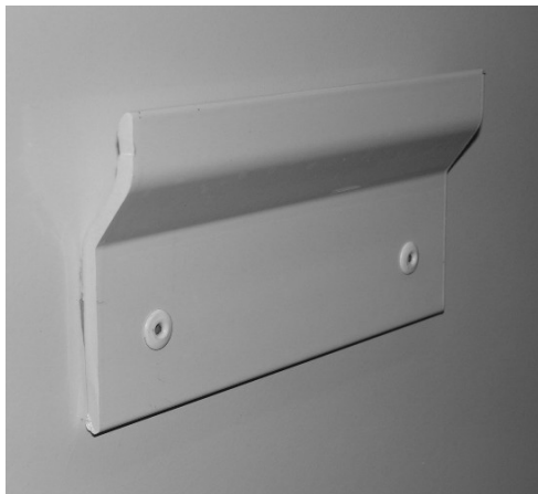
Bracket on Sidewall by Entrance Door
