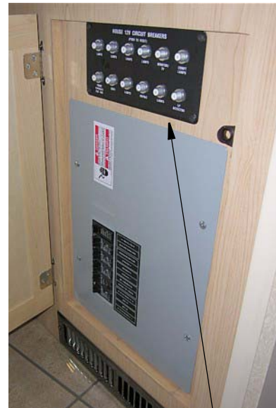
House 12-Volt Circuit Breaker Panel
