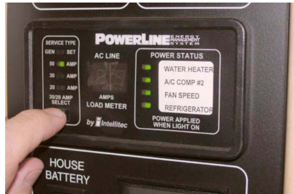
Energy Management System Display on Monitor Panel - Typical View
