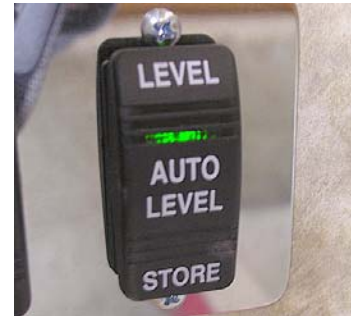
Auto Level Switch (Located inside entrance door)
