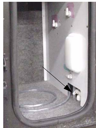
Waterline Drain Valve -Typical View
