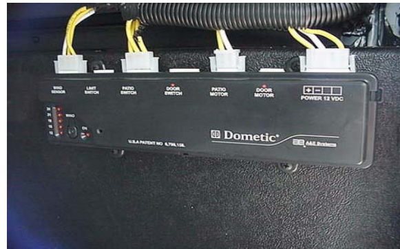
Awning Control Box (located in exterior compartment)
