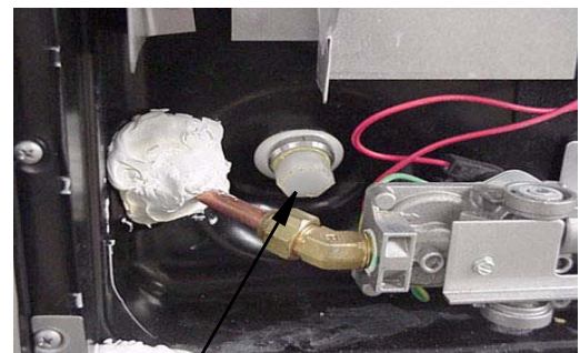
Water Heater Drain Plug (Remove with socket)
