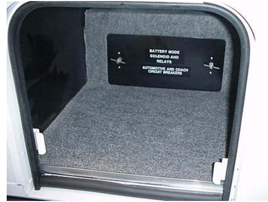
Chassis and House 12V Breakers in exterior storage compartment (remove cover to access)
