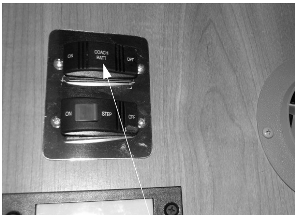
House/Coach Batt Disconnect Switch (Located near entrance door or end of galley, depending on model) -Typical View
