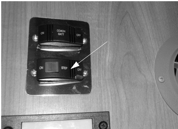
Entry Step Switch (Located near entrance door) -Typical View
