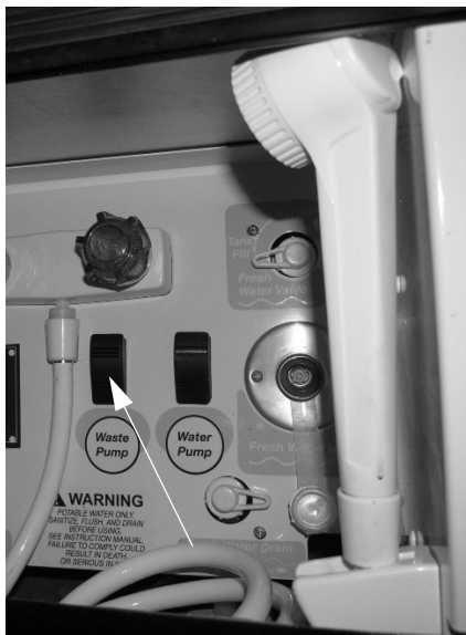
Waste Pump Switch (Located in water service center) -Typical View
