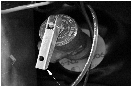
Pressure-Temperature Relief Valve (Lift handle only when water heater is cold)
