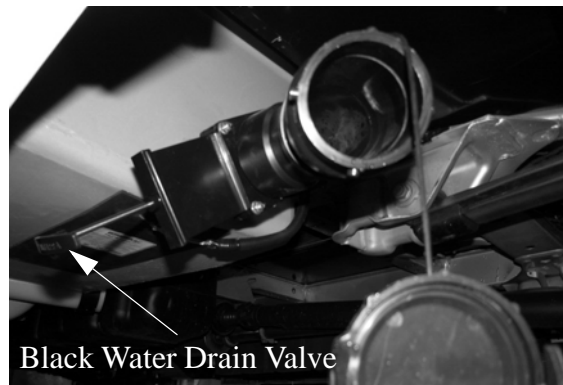
Black Water Drain Valve (Located ahead of rear driver side wheel) -Typical View
