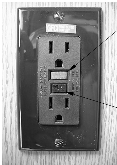
GFCI Outlet (Ground Fault Protector)
