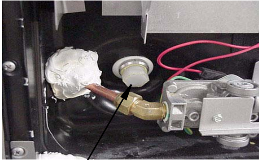
Water Heater Drain Plug (Remove with socket)
