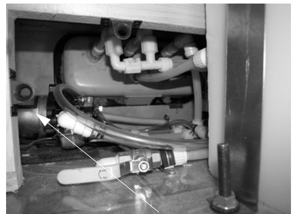
Water Pump (Located in backwall compartment - remove side panel to access) -Typical View
