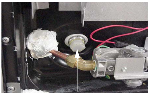
Water Heater Drain Plug (Remove with socket)
