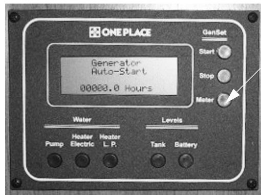
Generator Hourmeter Button -Typical View
