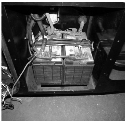
Chassis Batteries (Located in a rear driver side compartment) -Typical View
