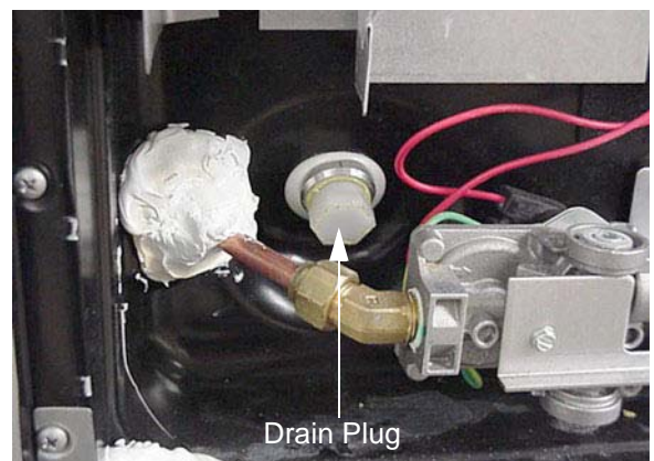
Water Heater Service Access -Typical View
