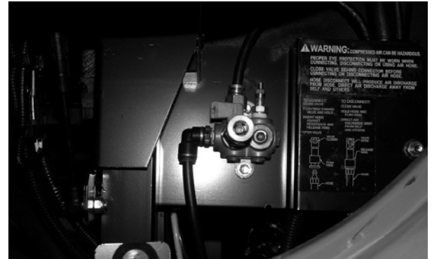
Quick Connect Air Coupler and Air Valve (Located behind front hood) -Typical View
