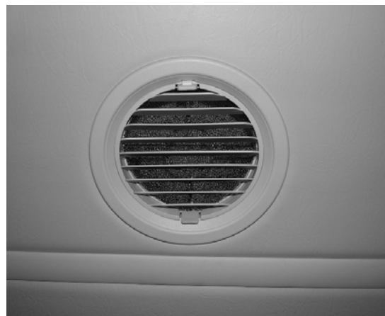
Return Air Vent (Shown with filter installed)
