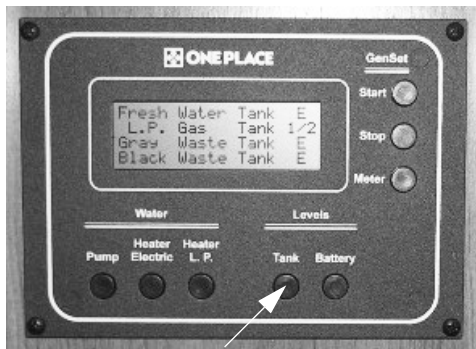
Tank Levels Switch
