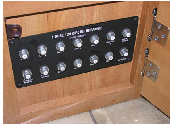
House Circuit Breakers -Typical View
