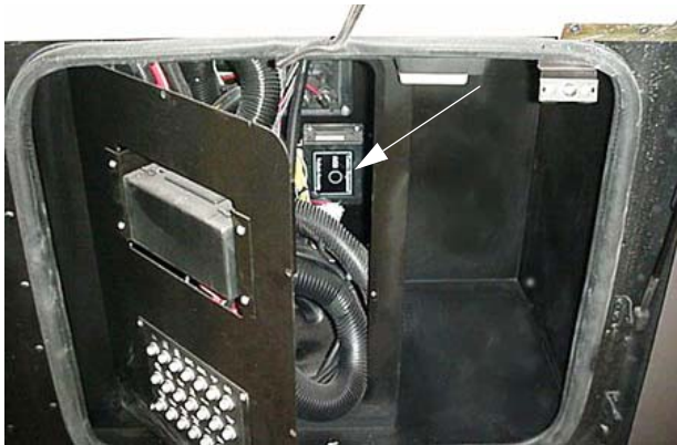
Keyless Entry Control Box (Located in 12-volt electrical compartment) -Typical View
