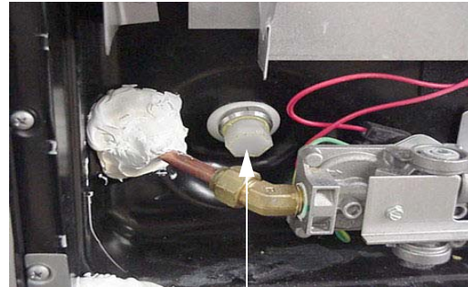
Water Heater Drain Plug (Remove with socket)
