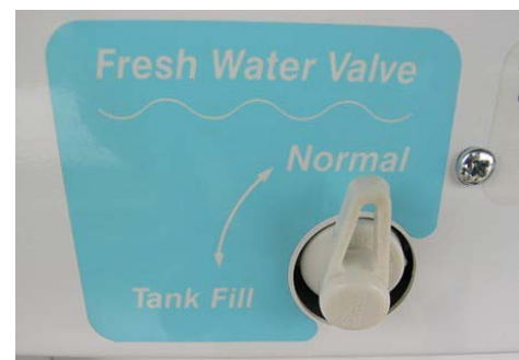
Fresh Water Valve in Normal use position (located inside the exterior wash station)
