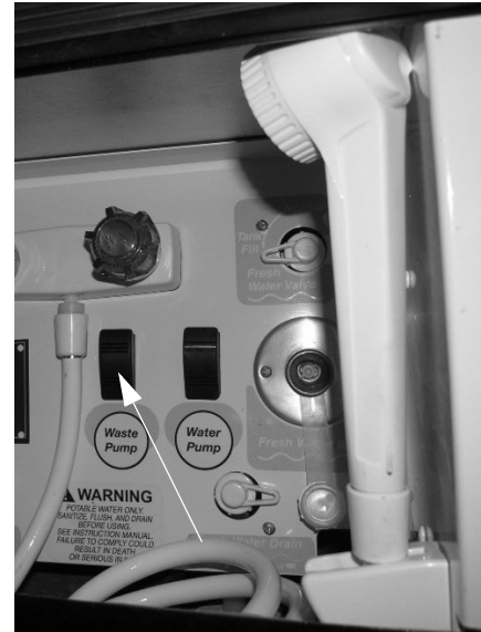
Waste Pump Switch (Located in water service center) -Typical View
