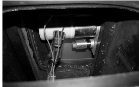
Front Slideout Motor/Gearbox (Close-up view from opening above sewage drain hose) -Typical View
