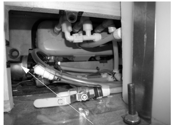
Water Pump (Located in backwall compartment - remove side panel to access) -Typical View
