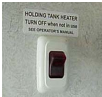
Holding Tank Heater Switch (Located near monitor panel) -Typical View
