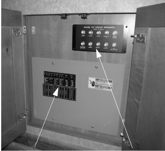
120-Volt House Circuit Breakers
