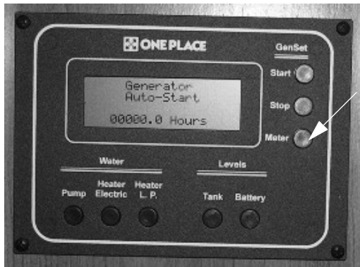
Generator Hourmeter Button -Typical View
