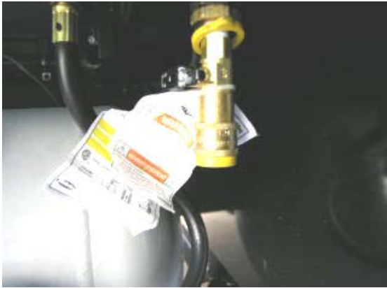
LP Accessory Connection (Located behind LP Tank access door on passenger side of coach) -Typical View
