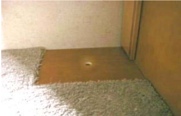
Water Supply Faucets (Located behind access door in the wardrobe floor.)
