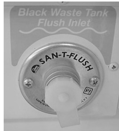
Black Waste Tank Flush Inlet (Located in water service center) -Typical View
