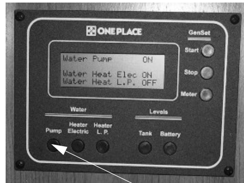
Water Pump Switch
