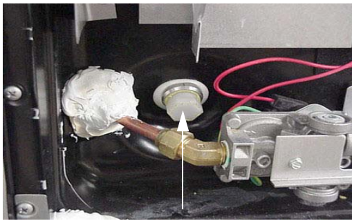
Water Heater Drain Plug (Remove with socket)
