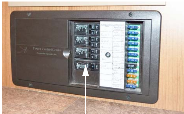
120-Volt Circuit Breakers -Typical View
