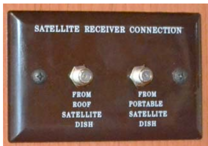
Interior Connection for Satellite Dish (Located near entertainment center cabinet)
