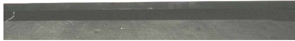
Holding Tank Dump Valves (Located in mid-driver side access compartment) -Typical View
