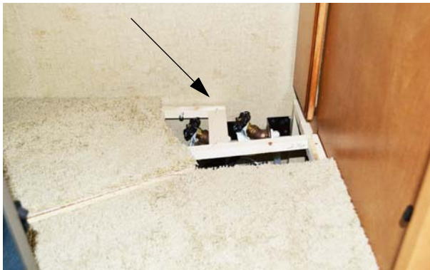
Water Supply Faucets (Located beneath access door in the wardrobe floor.)
