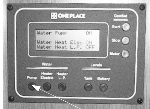
Water Pump Switch
