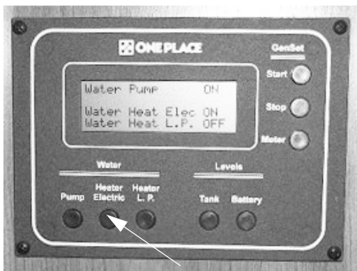
Electric Water Heater Switch (Located on OnePlace monitor panel)
