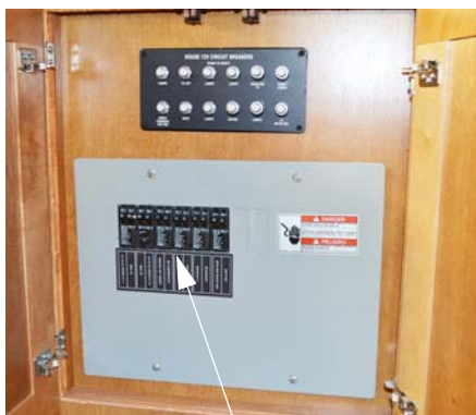
120-Volt House Circuit Breakers -Typical View
