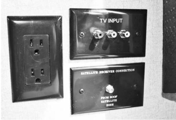
Bedroom DVD/Satellite Receiver Connection -Typical View
