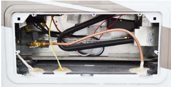
Refrigerator Access Compartment -Typical View
