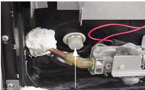
Water Heater Drain Plug (Remove with socket)
