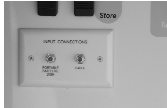
Exterior Connections for Cable TV and Satellite Dish (Located in water service center) -Typical View
