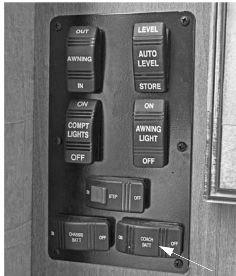
House/Coach Battery Disconnect Switch (Located near entrance door) -Typical View
