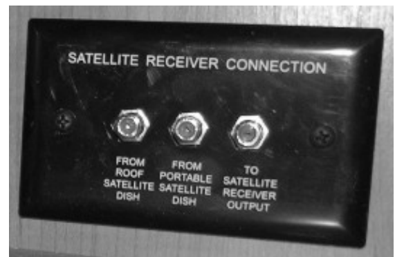
Interior Connection for Satellite Dish (Located in a cabinet near TV) -Typical View
