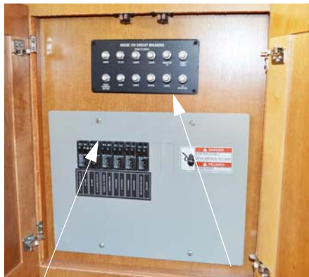
120-Volt House Circuit Breakers
