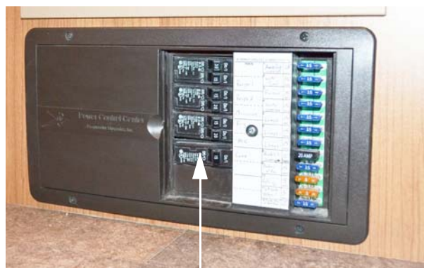
120-Volt Circuit Breakers -Typical View
