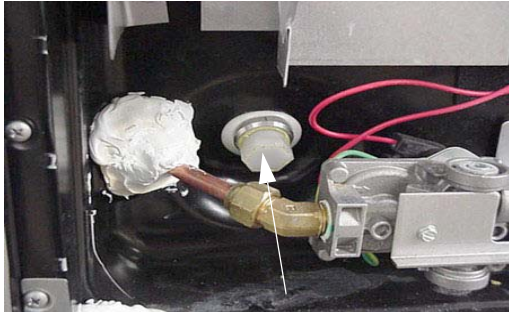
Water Heater Drain Plug (Remove with socket)
