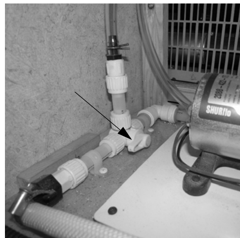
Winterization Valve -Typical View
