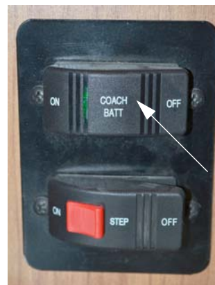
House/Coach Battery Disconnect Switch (Located near entrance door or end of galley, depending on model) -Typical View
