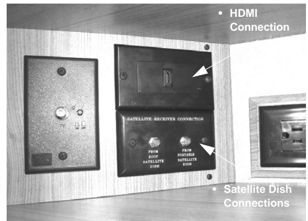
Interior Satellite Dish and HDMI Connections (Located near entertainment center cabinet) -Typical installation shown
