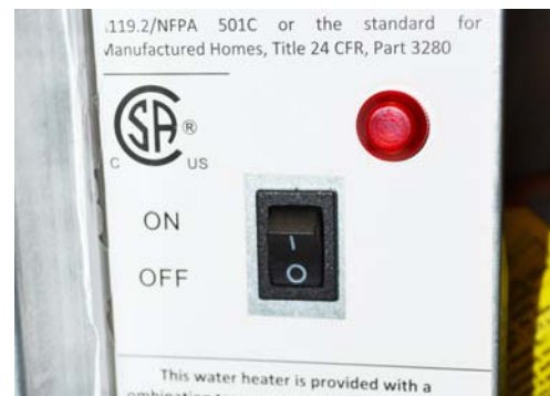
Water Heater (Tankless) Power Switch
