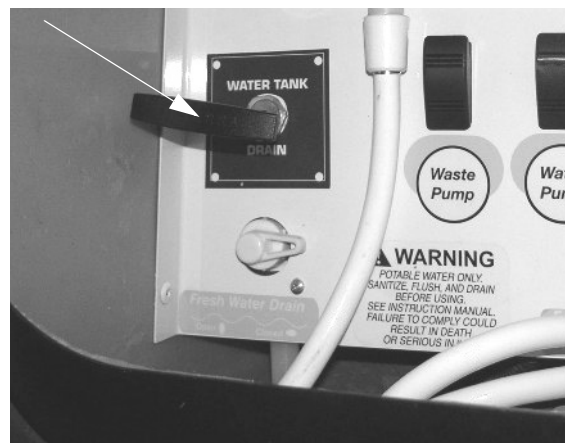
Water Tank Drain Valve -Typical installation shown
