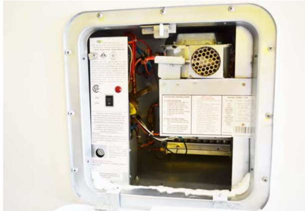
Water Heater Exterior Service Access -Typical View
