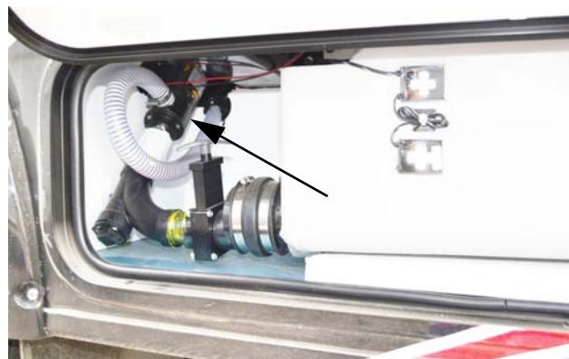
Waste Pump (Located in driver side compartment behind rear wheel)
