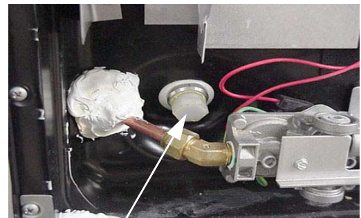
Water Heater Drain Plug (Remove with socket)
