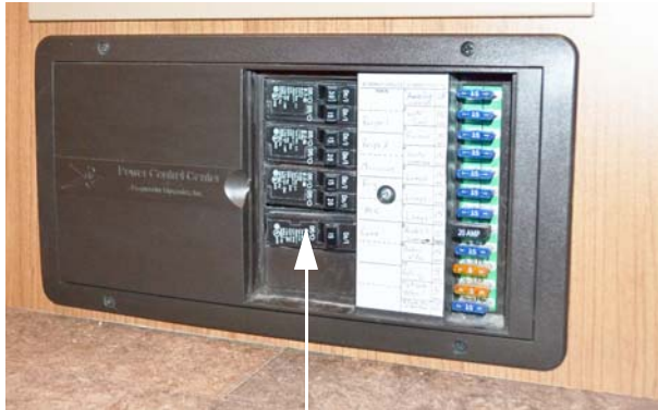
120-Volt Circuit Breakers -Typical View
