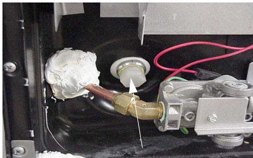
Water Heater Drain Plug (Remove with socket)
