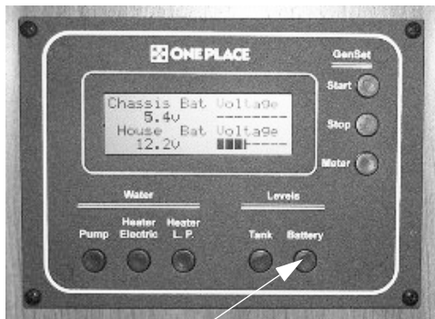
Battery Levels Switch
