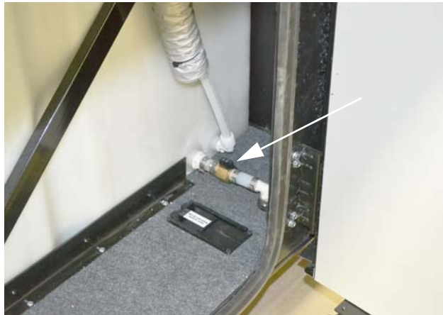
Water Tank Drain Valve (Located in the third passenger side compartment) -Typical View
