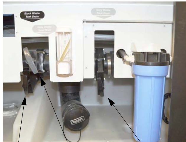
Black Waste Tank Drain Valve
