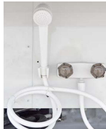
Exterior Shower/Wash Station -Typical View
