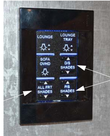
12-Volt Night Shade Switches - Lounge *Switch located by sofa shown -Typical View
