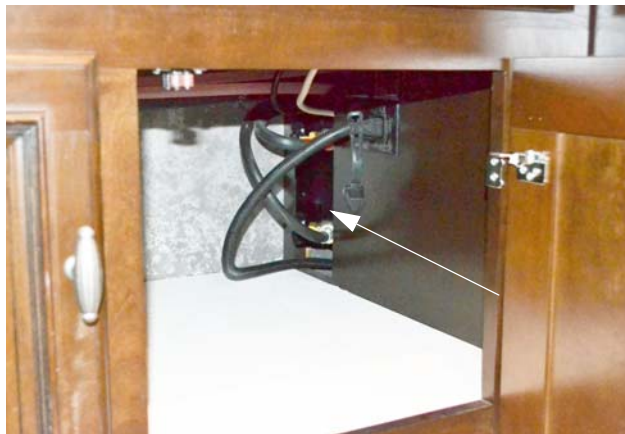
Water Supply Faucets (Located below lavatory cabinet) -Typical View
