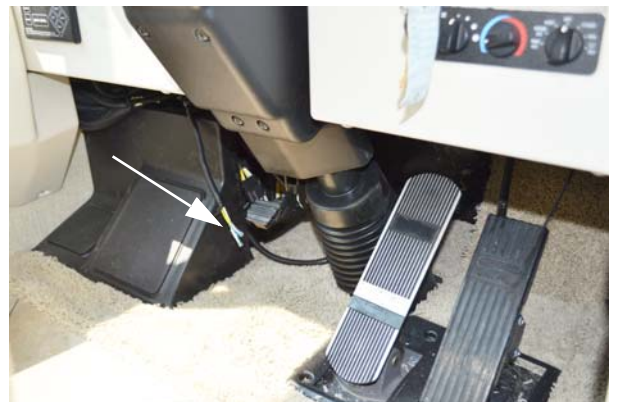
CB Power Wires -Typical View
