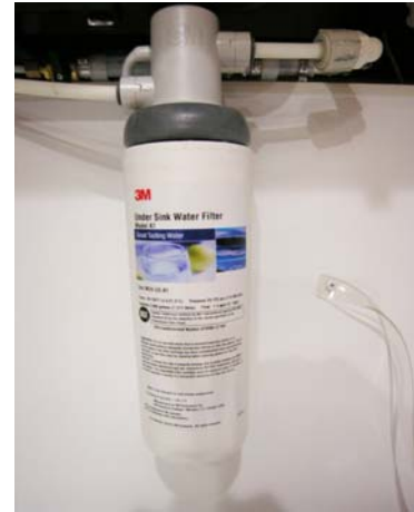
Cold Water Filter Assembly (Located below galley sink)
