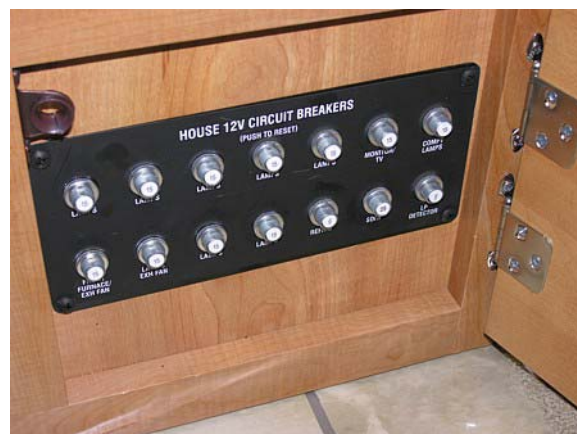
House Circuit Breakers -Typical View
