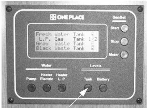
Tank Levels Switch
