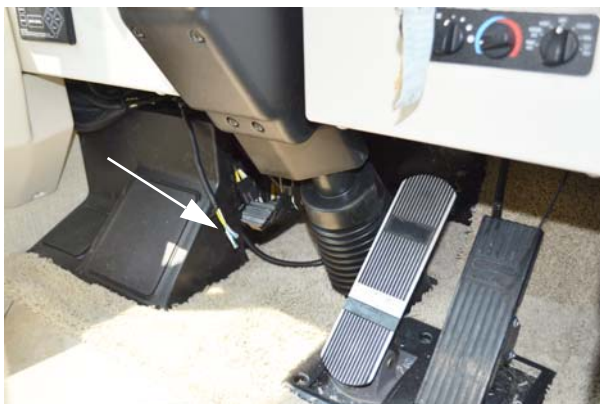
CB Power Wires -Typical View
