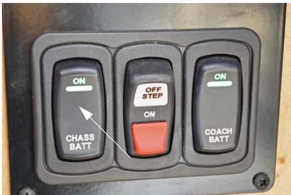
Chassis Battery Disconnect Switch (Located near entrance door) -Typical View
