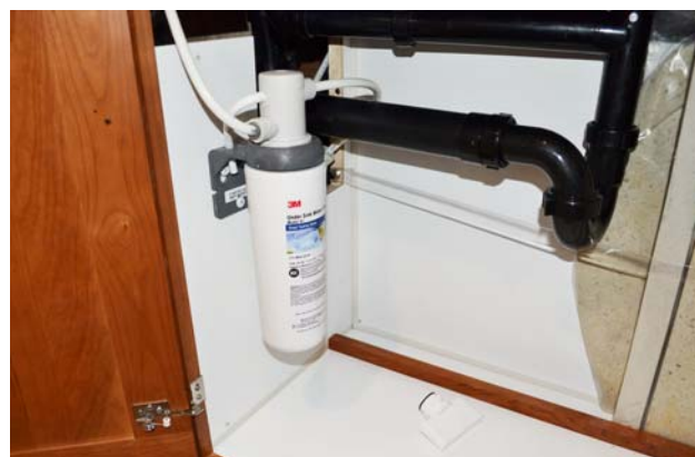
Galley Filtered Cold Water Faucet/ Ice Maker Filter Assembly (Located below galley sink) -Typical View
