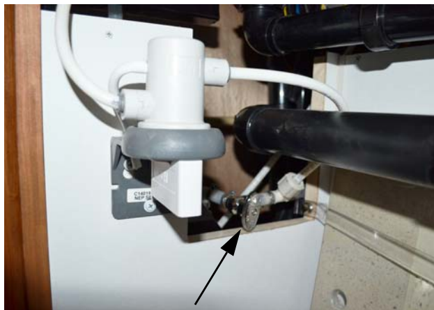
Pot Filler and Ice Maker Water Supply Valve (Located below galley sink) -Typical View
