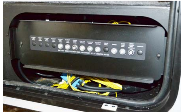
Automotive Chassis and House 12-Volt Circuit Breakers (Located inside passenger compartment) -Typical View
