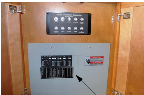
120-Volt House Circuit Breakers -Typical View
