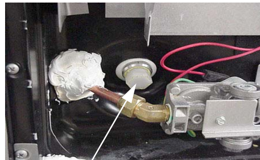
Water Heater Drain Plug (Remove with socket)
