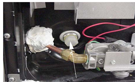
Water Heater Drain Plug (Remove with socket)
