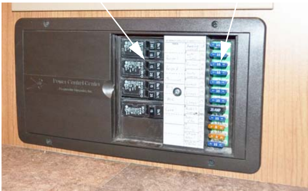
Power Center (Converter) -Typical View
