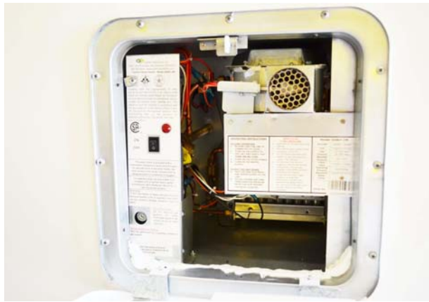
Water Heater Exterior Service Access -Typical View
