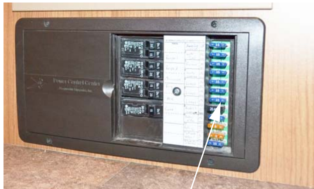
House 12-Volt Fuses (Located on the right-hand side of the power converter) -Typical View
