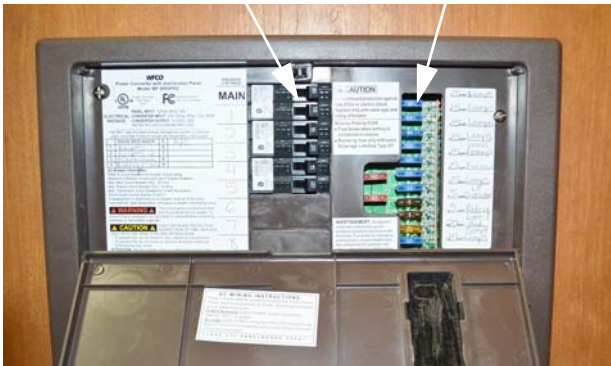
Power Center (Converter) -Typical View
