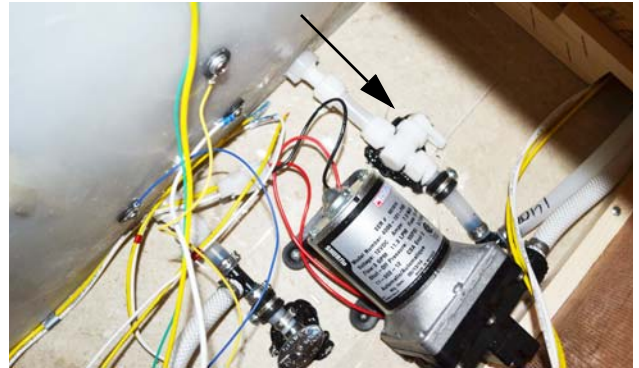
Waterline Drain Valve -Typical View
