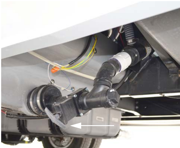
Gray Waste Tank Drain Valve (Located beneath driver side of coach ahead of rear wheel) -Typical View
