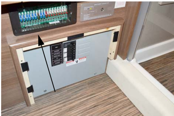
House 12-Volt Fuses (Located on right side twin bed cabinet at rear) -Typical View
