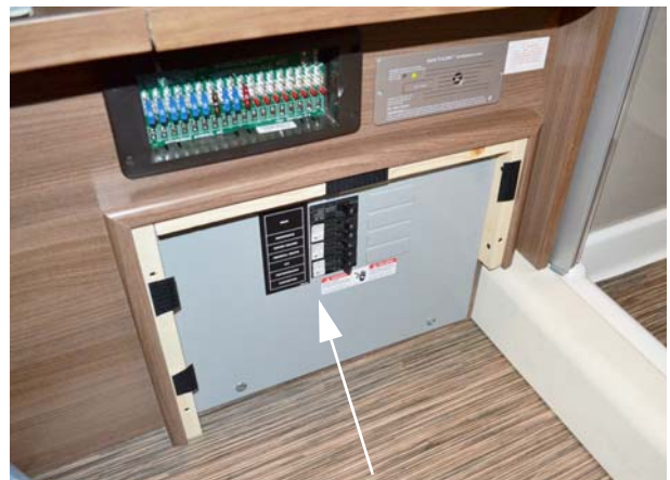
120-Volt Circuit Breakers -Typical View
