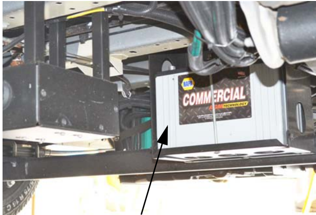
House Battery Access (Located behind rear tires) - Remove bolts from battery retainer to remove house battery
