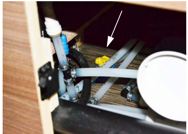
Water Heater Drain Valve
