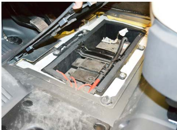
Chassis Batteries Access (Located beneath driver side floor mat) -Typical View
