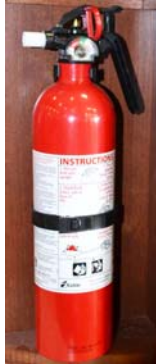
Fire Extinguisher (Located near sliding entrance door)
