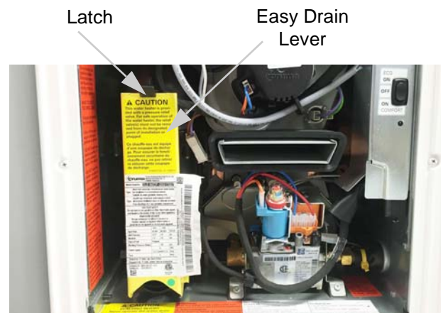
Easy Drain Lever (Located behind water heater access panel on exterior of coach)
