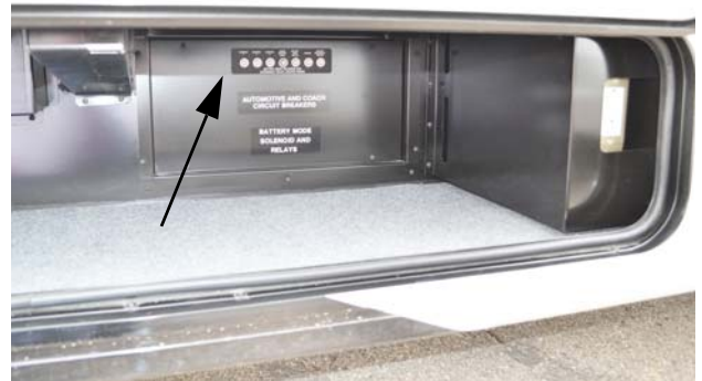
Automotive Chassis and House 12-Volt Circuit Breakers (Located inside passenger compartment) -Typical View
