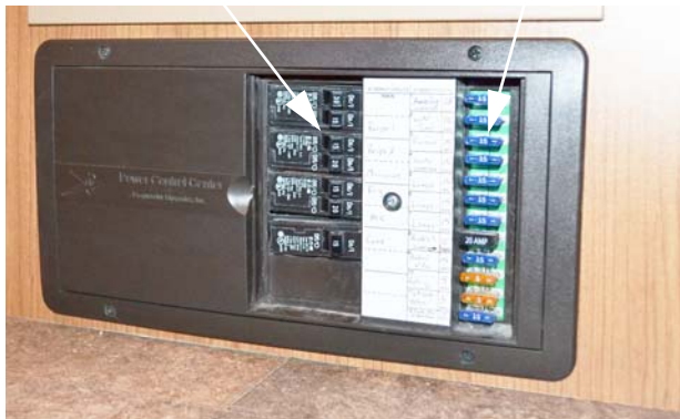
Power Center (Converter) -Typical View
