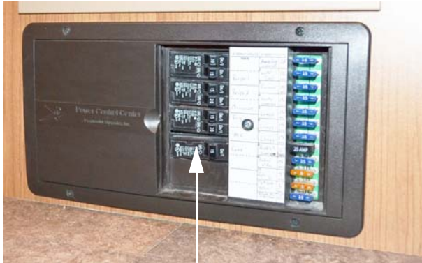
120-Volt Circuit Breakers -Typical View
