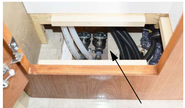
Waterline Drain Valves -Typical installation shown
