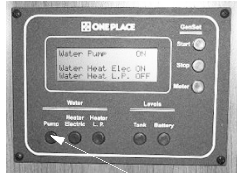
Water Pump Switch
