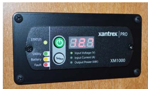
Inverter Control Panel (Located near monitor panel) -Typical View
