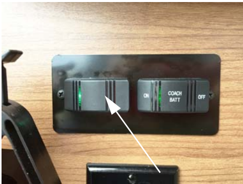
Accent LED Running Board Light Switch (Located near sliding door) -Typical View
