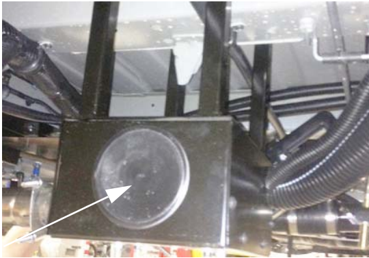
Waste Pump Enclosure (Located beneath coach)
