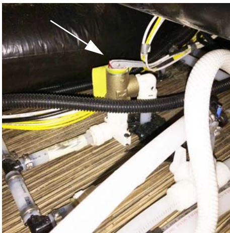
Pressure Temperature Relief Valve (Lift handle only when water heater is cold)
