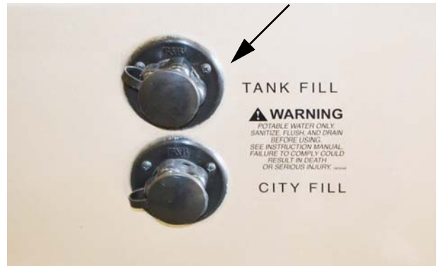
Tank Fill Inlet (Located on the left sidewall) -Typical View
