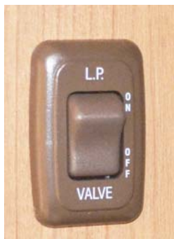
LP Tank Valve Switch
