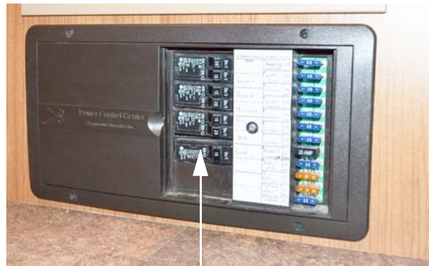
120-Volt Circuit Breakers -Typical View
