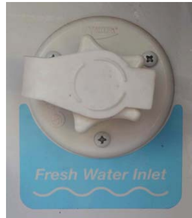
Fresh (City) Water Connection “Fresh Water Inlet” (Located in the water service center) -Typical View
