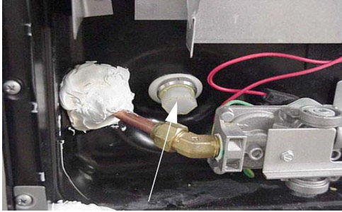
Water Heater Drain Plug (Remove with socket)
