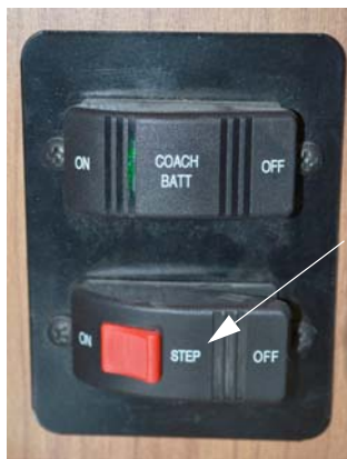
Entry Step Switch (Located near entrance door) -Typical View
