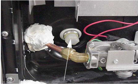
Water Heater Drain Plug (Remove with socket)
