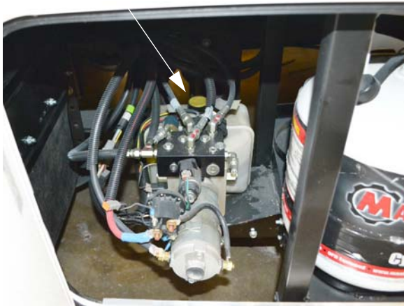
Hydraulic Oil Reservoir (Located behind driver side front tire) -Typical View
