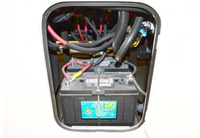
House/Coach Batteries -Typical View
