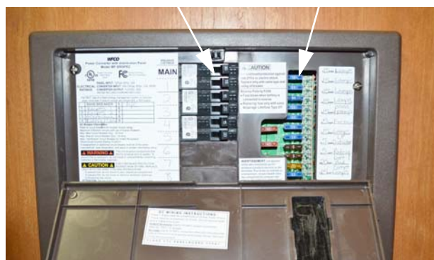
Power Center (Converter) -Typical View
