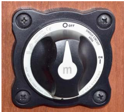
House/Coach Battery Disconnect Switch (Located an exterior compartment near the entrance door) -Typical View
