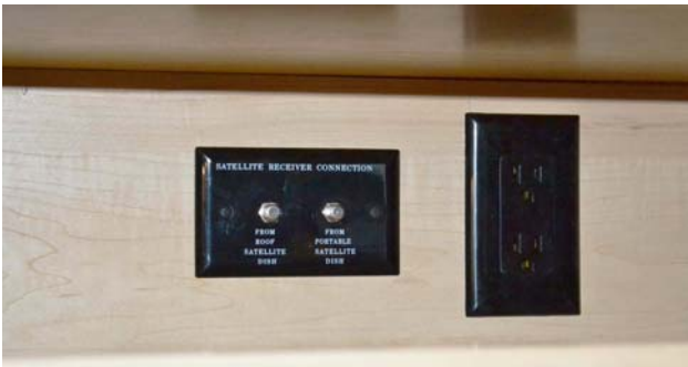
Interior Connection for Satellite Dish (Located in cabinet behind front overhead TV) -Typical View
