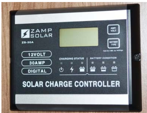
Solar Charge Controller (Located near monitor panel)
