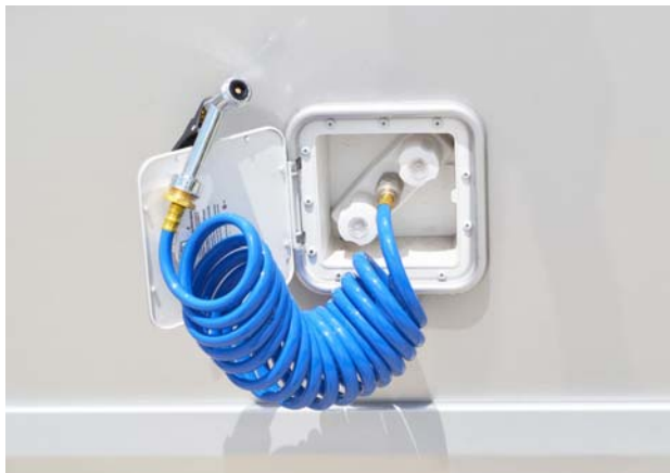
Exterior Shower/Wash Station (Typical)
