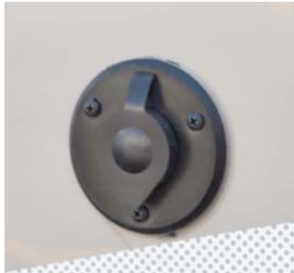
Exterior TV Connection (Located near entrance door) -Typical View
