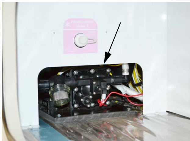
Water Pump • Model 23A - located inside a passenger side compartment -Typical View
