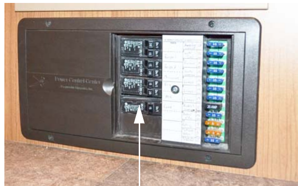
120-Volt Circuit Breakers -Typical View
