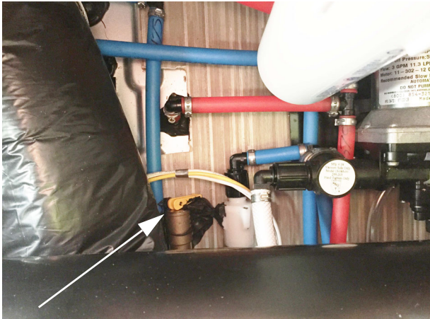
Water Heater Drain (Yellow) Valve
