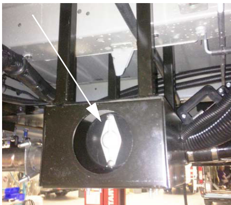
Waste Pump (Located beneath motorhome)
