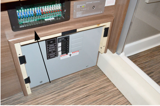
House 12-Volt Fuses (Located near the bed) -Typical View
