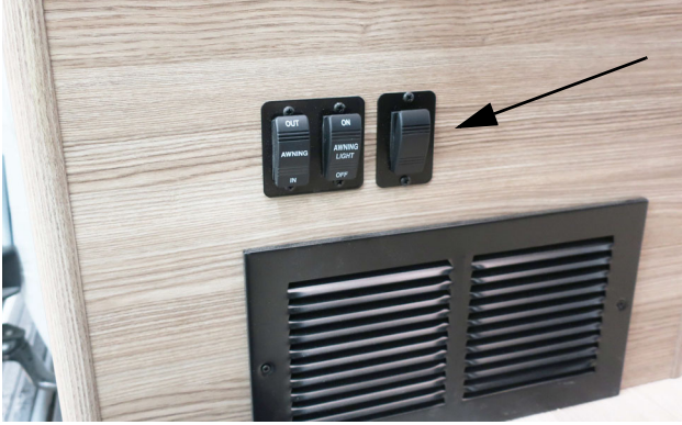
Accent LED Running Board Light Switch (Located near sliding entrance door) -Typical View
