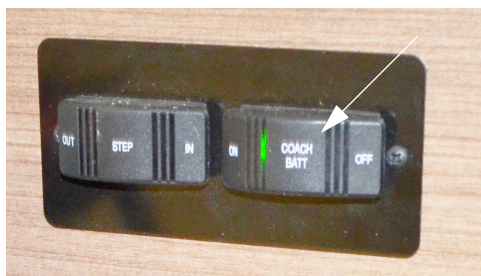
House/Coach Battery Disconnect Switch (Located near sliding door)
