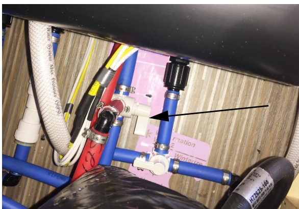
Winterization Valve 1 (Water Heater Bypass Valve) (See “Water System Drain Valve Locations” chart at the end of this section for location on your model) *Model 59K shown
