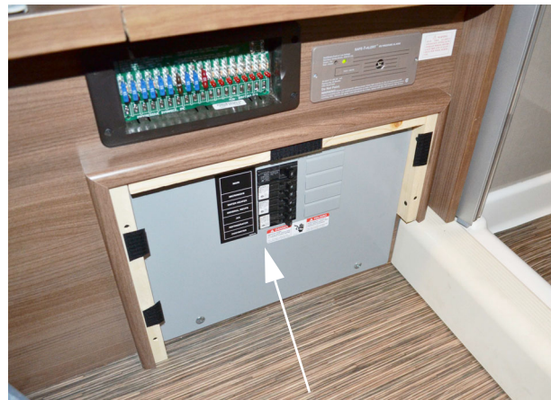
120-Volt Circuit Breakers -Typical View
