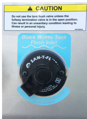
Black Waste Tank Flush Inlet (Located on right sidewall)
