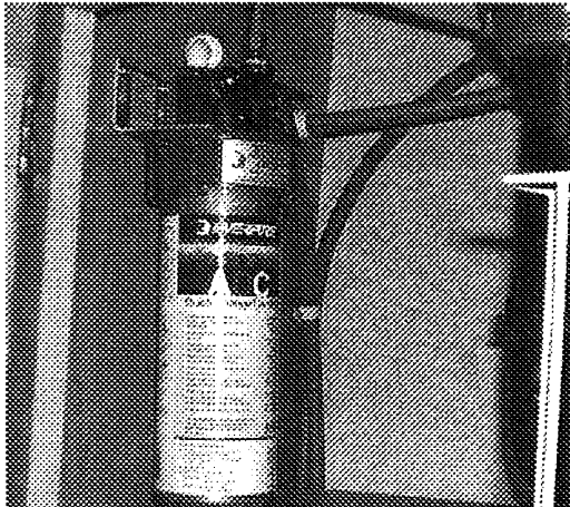
Water Filter Assembly - Below Galley Sink
