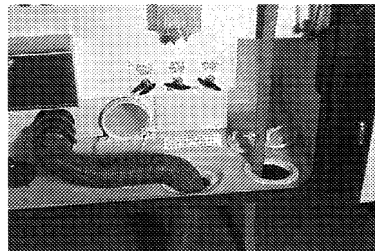
Drainage Hose & City Water Hose routed through passages in compartment
