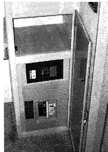
House 110-Volt Breaker Panel in bedroom wardrobe cabinet
