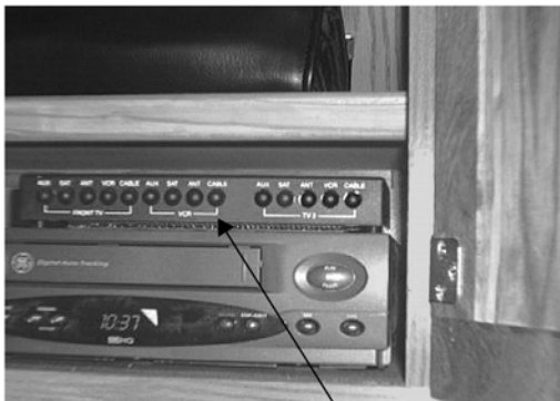
Video Selector System (in right front overhead compartment)
