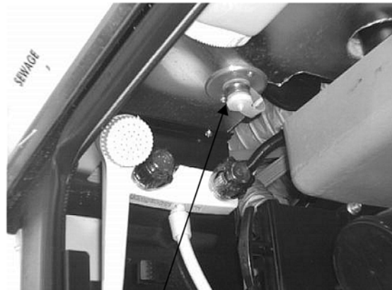
City Water Connection
