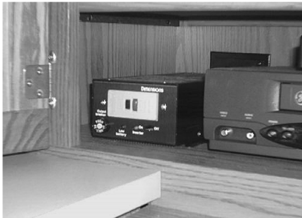
DC-AC Voltage Inverter in Video Center
