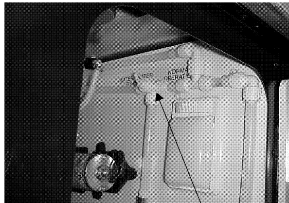
Water Heater Bypass Valve
