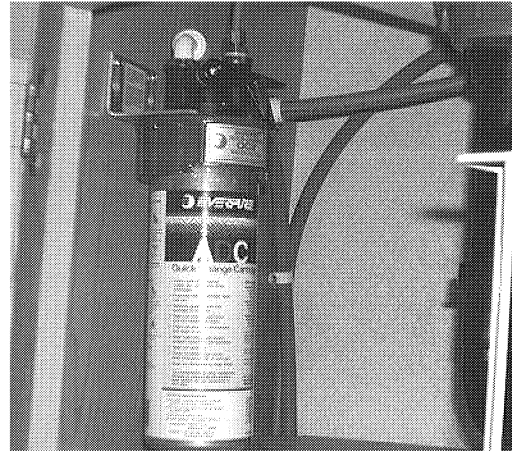
Water Filter Assembly - Below Galley Sink
