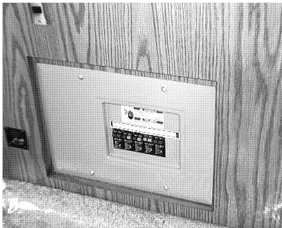
House 110-volt Breaker Panel
