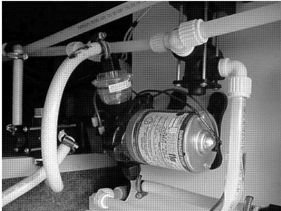
Water Pump and Filter
