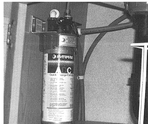
Water Filter Assembly - Below Galley Sink
