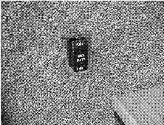
Aux. Batt. Disconnect Switch in Entrance Stepwell
