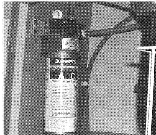
Water Filter Assembly - Below Galley Sink
