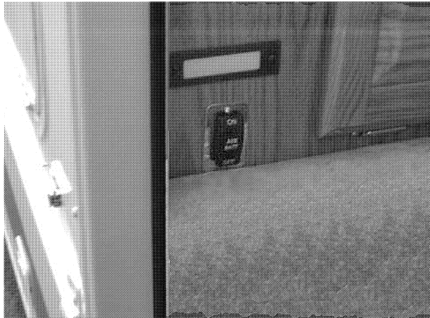
Aux. Batt. Switch (Near entrance door)
