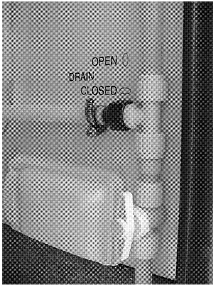
Water Line Drain Valve
