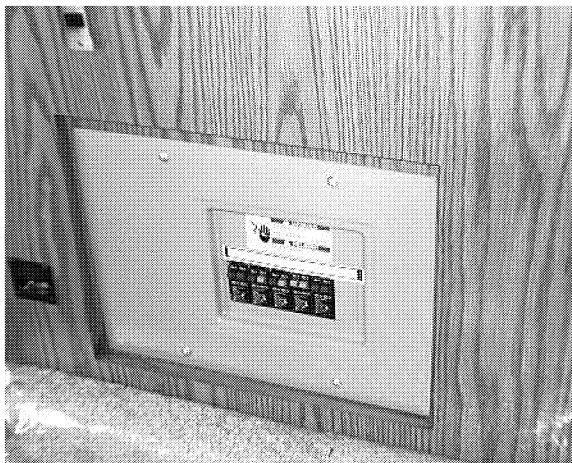
House 110-volt Breaker Panel
