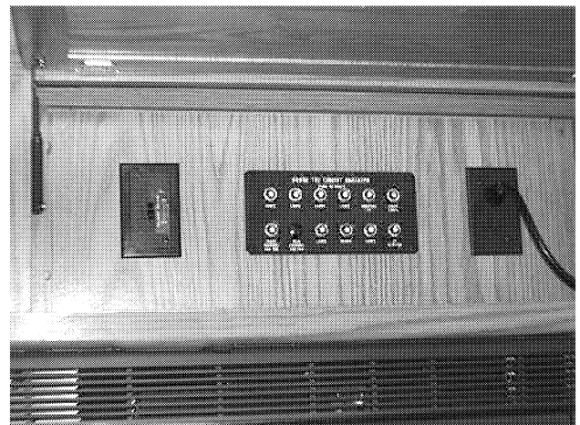
House 12-Volt Breaker Panel
