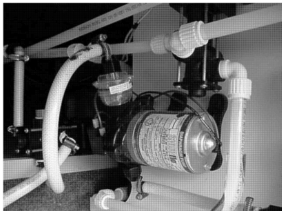
Water Pump and Filter
