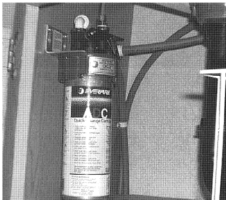
Water Filter Assembly - Below Galley Sink
