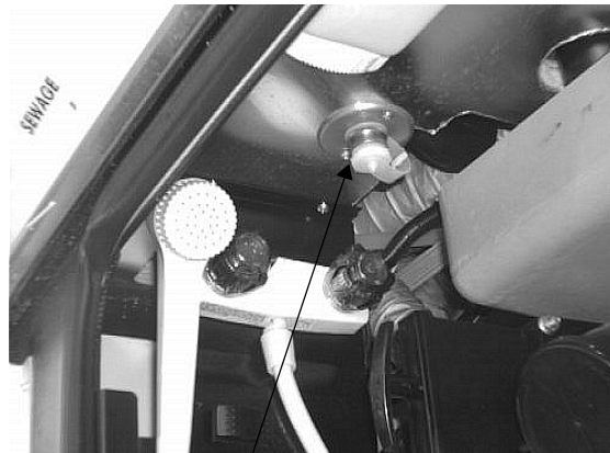
City Water Connection
