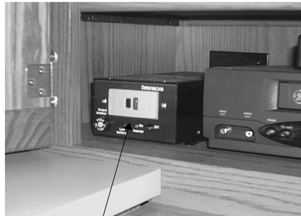
DC-AC Voltage Inverter in Video Center
