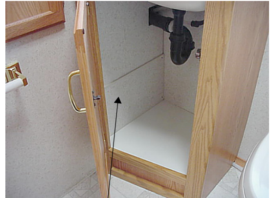
Water Heater Bypass Valve and Winterization Siphon Valve behind Access Panel beneath Bath Lavatory Vanity
