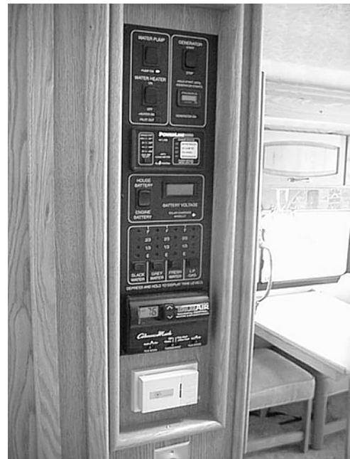
One Place Monitor Panel
