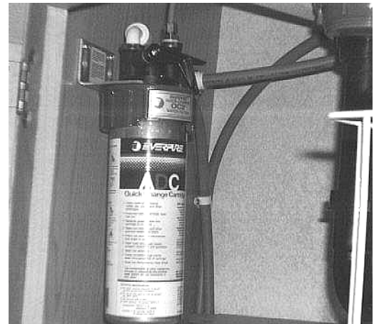
Water Filter Assembly - Below Galley Sink
