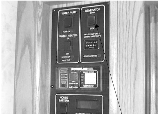
Generator Switch and Hourmeter
