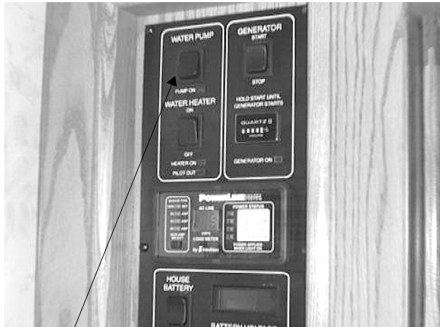
Water Pump Switch
