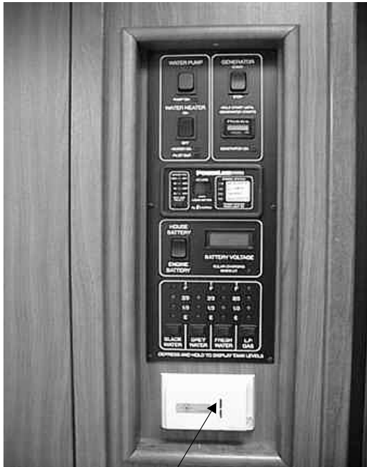
Power Vent Thermostat Bath Area
