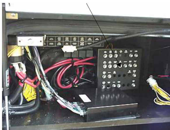
Automotive/Chassis Electrical Center (Left Front Compartment)
