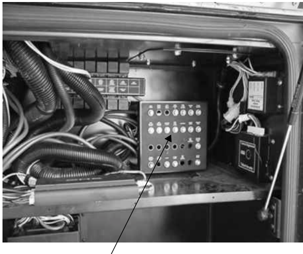
Automotive 12-Volt Breaker Panel
