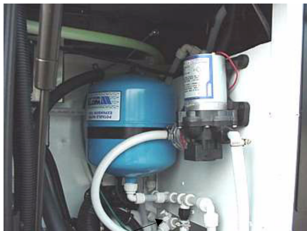
Water Line Drain Valves (in water pump compartment)
