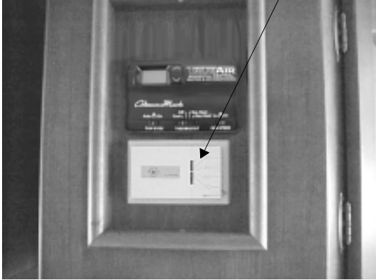
Power Ventilator Thermostat - Galley
