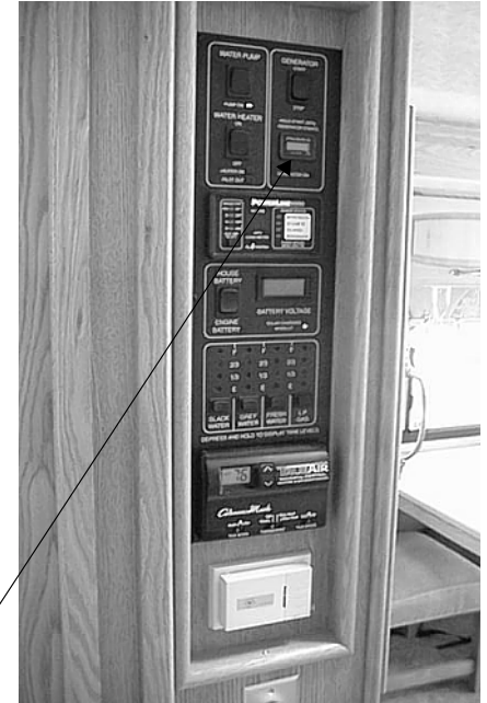
Generator Switch and Hourmeter
