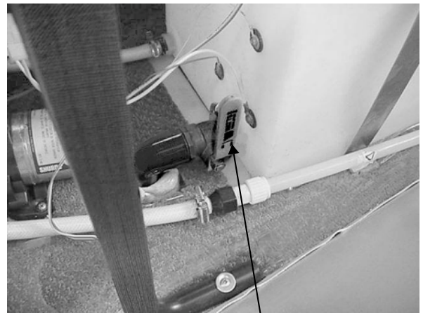
Water Tank Drain Valve
