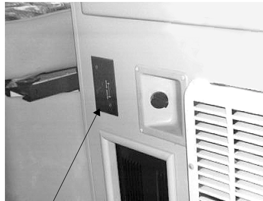
Water Heater Power Switch
