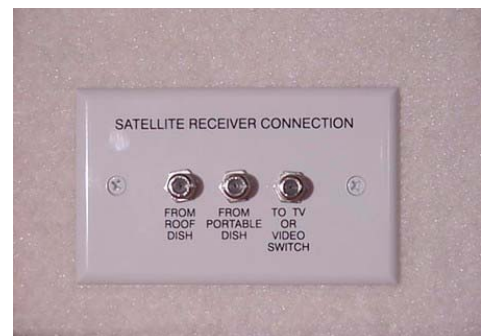
Interior Connection for Satellite Dishes (in front video center cabinet)
