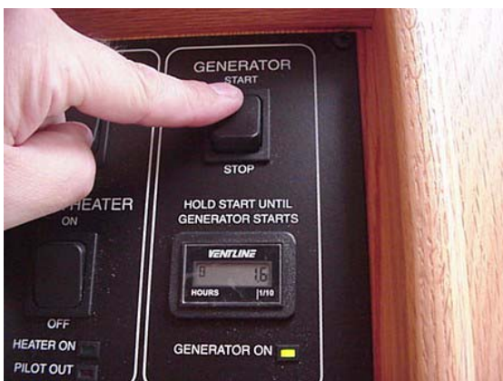
Generator Switch and Hourmeter
