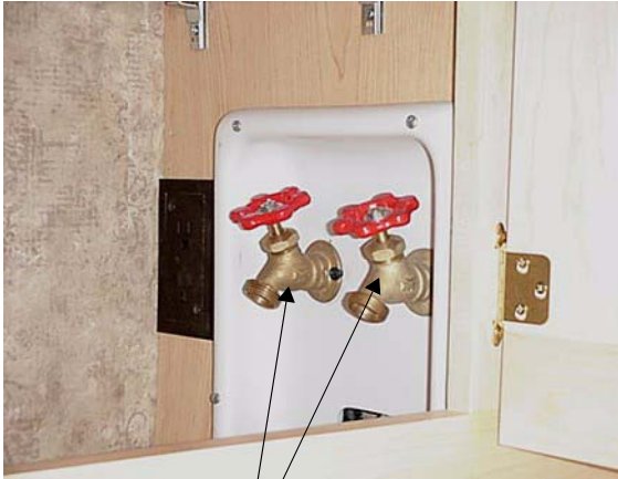
Water Supply Faucets Typical
