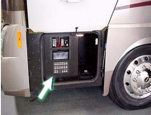
12V Electrical Compartment
