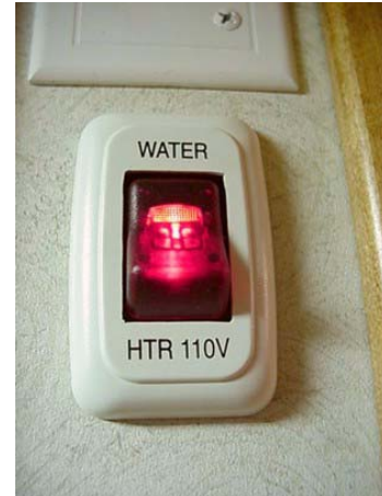
Electric Water Heater Switch (Typical)
