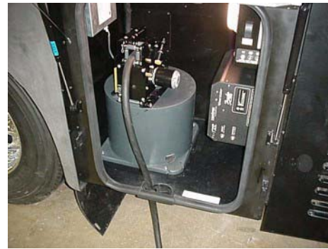
Inverter Charger Unit Location in shoreline compartment
