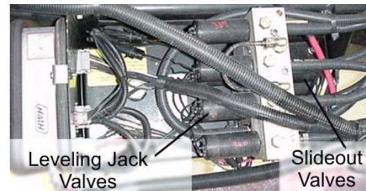
Slideout Pump beneath Entry Step
