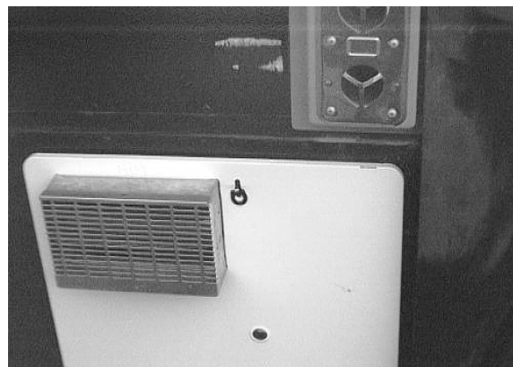
Water Heater Service Access Panel
