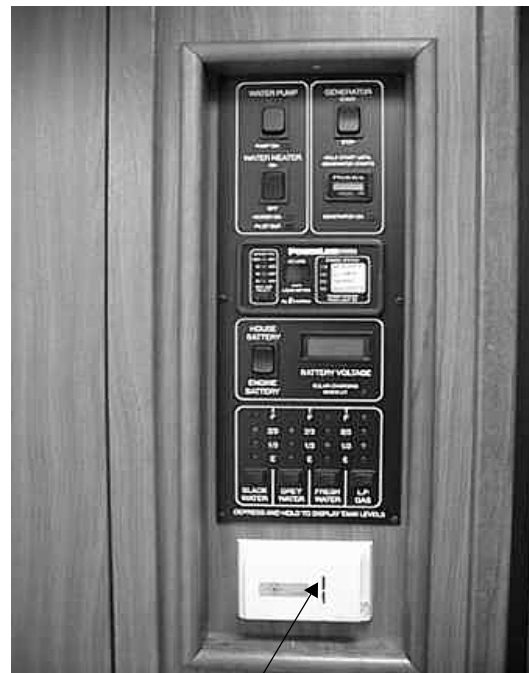
Power Vent Thermostat Bath Area
