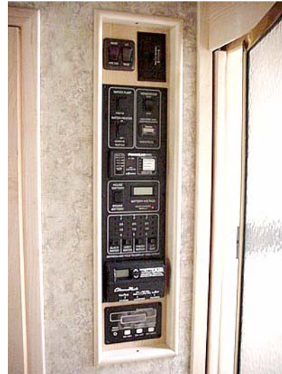
One Place Monitor Panel
