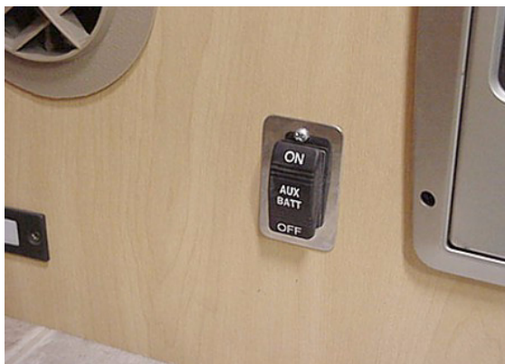
Aux. Batt. Switch (Near entrance door)
