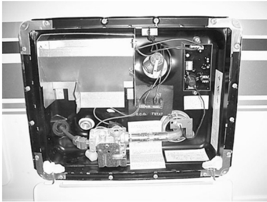
Water Heater Exterior Service Access
