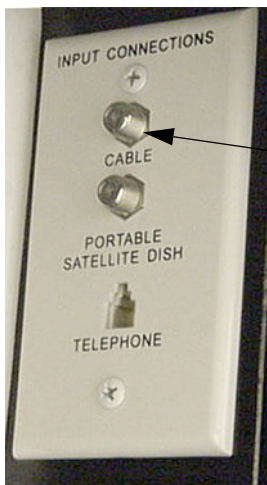
Exterior Connection for Cable TV (In Water Center Compartment)
