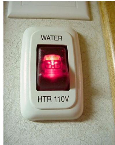
Electric Water Heater Switch (Typical)
