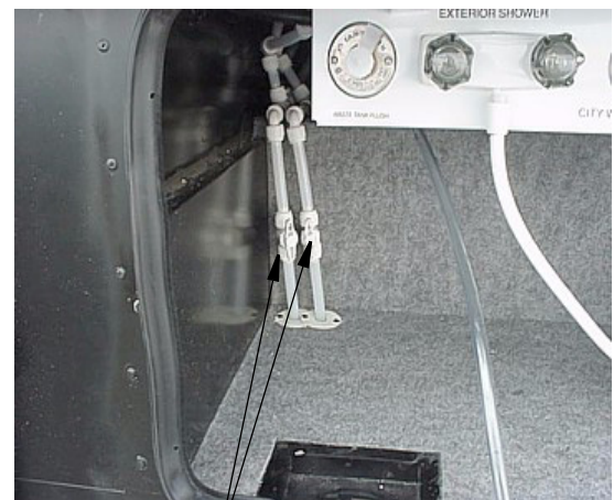
Water Drain Valves in Water Center (Model 430V)
