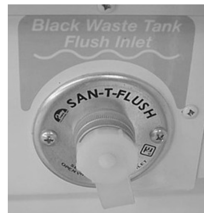
Black Water Tank Flush Inlet (Located in water service center) -Typical View
