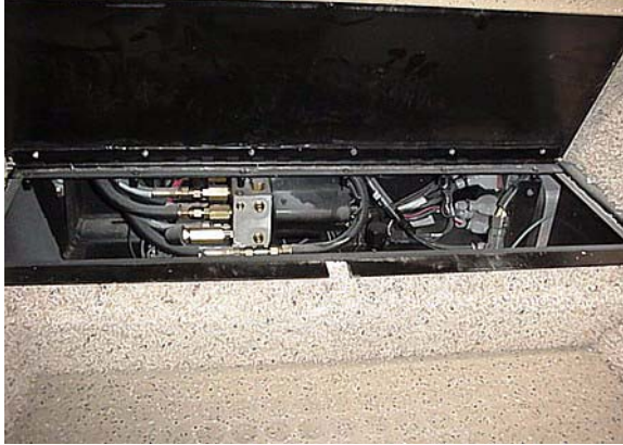
Hydraulic Pump beneath Entry Step
