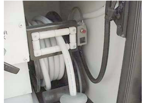
Water Hose Reel
