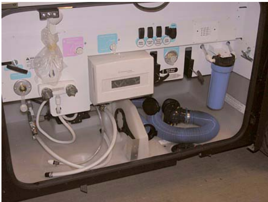
Water Service Center - typical view
