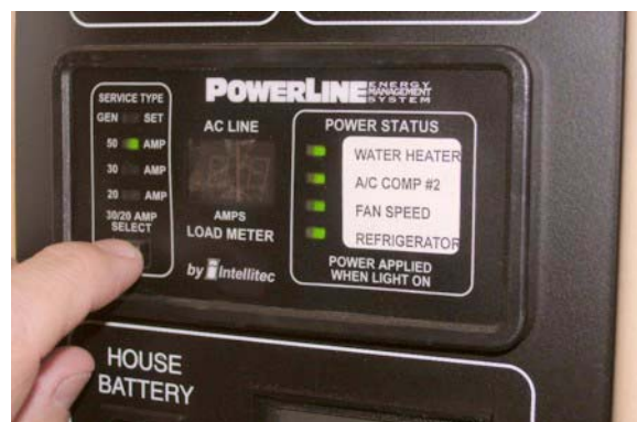
PowerLine EMS Display on Monitor Panel - typical
