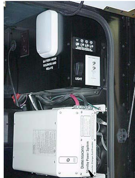
Inverter Charger Unit Location in utility compartment
