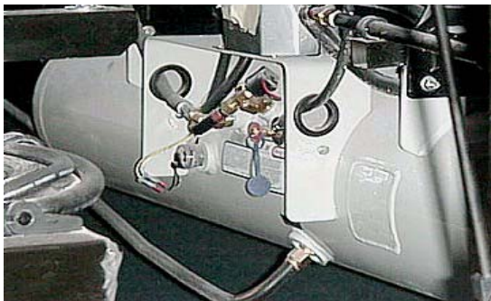
Propane Gas Tank behind slideout room
