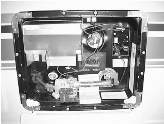
Water Heater Exterior Service Access
