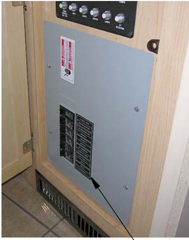
120-Volt House Circuit Breakers - typical
