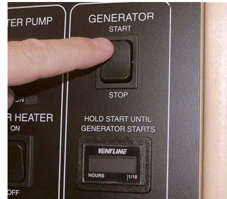
Generator Switch and Hourmeter on monitor panel
