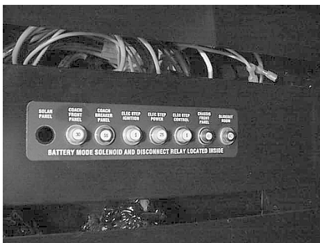
Auto Chassis 12-Volt Circuit Breaker Panel (cover removed)
