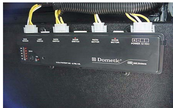
Awning Control Box (located in exterior compartment)
