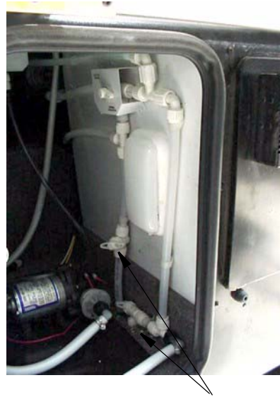
Water Line Drain Valves
