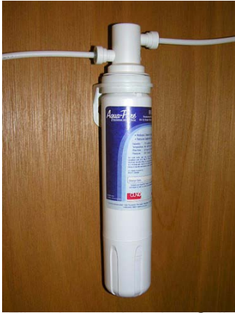
Water Filter Assembly below Galley Sink
