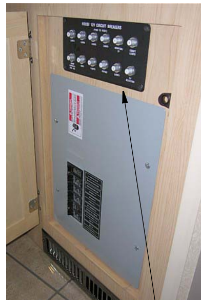
House 12-Volt Circuit Breaker Panel
