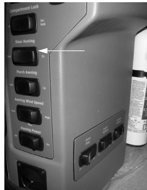
Over the Door Awning Switch - Typical View (Located near the entrance door)
