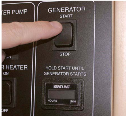
Generator Switch and Hourmeter
