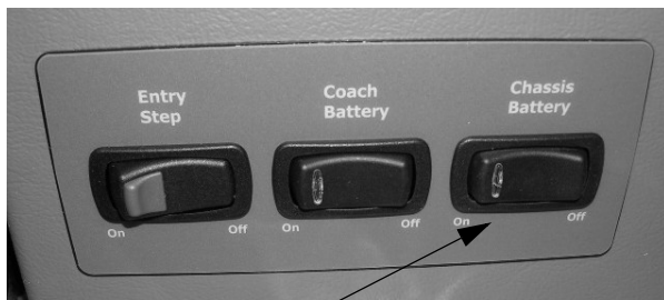
Chassis Battery Disconnect Switch (located inside the entrance door)
