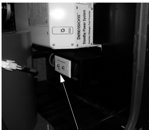
Exterior Input Connections for Satellite Dish and Cable TV (in Water Center or Utility Compartment)
