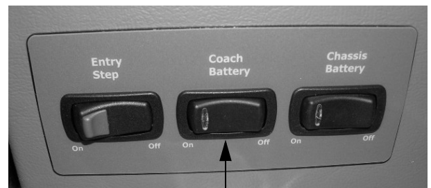
Aux. Battery Disconnect Switch (Near Entrance Door)
