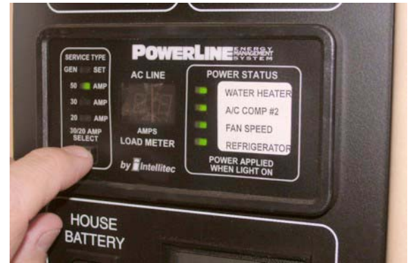
Energy Management System Display on Monitor Panel - Typical View
