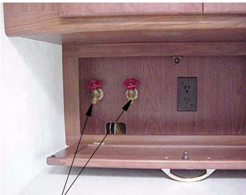
Water Supply Faucets - Typical
