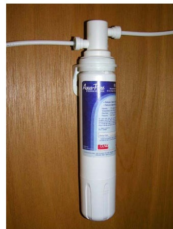
Water Filter Assembly below Galley Sink
