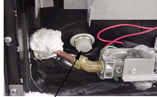
Water Heater Drain Plug Remove with socket
