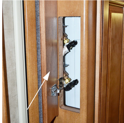
Water Supply Faucets (Located behind access door rear of the washer/dryer cabinet.)
