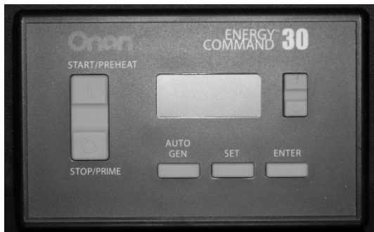
AGS Control Pad (Located near monitor panel)
