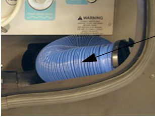
Sewage Drain Hose -Typical View
