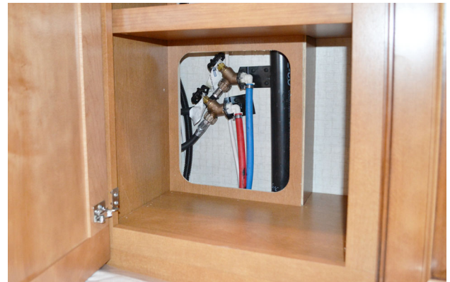
Water Supply Faucets (Located inside cabinet front of washer/dryer - remove access panel)
