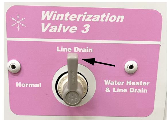
Winterization valve in the “Line drain” position. -Typical View
