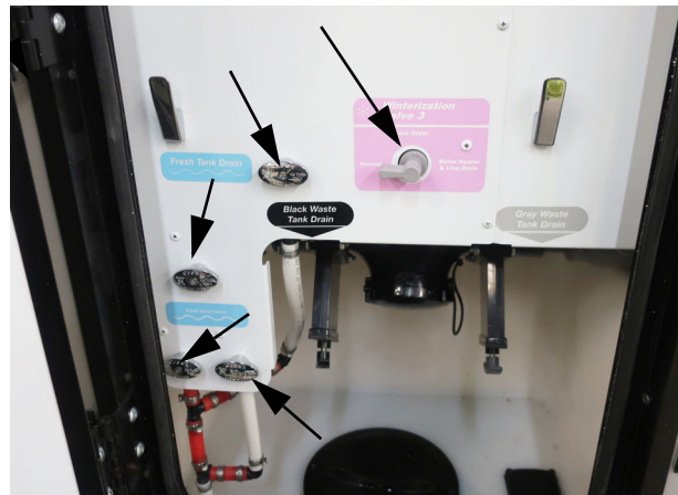
Waterlines and Tank Drain Valves (Shown in the closed position) -Typical View
