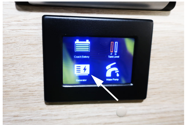
Generator location on the main screen of the Systems Monitor Panel -Typical View
