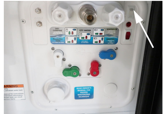
Water Pump Switch on the Water Center Panel. -Typical View
