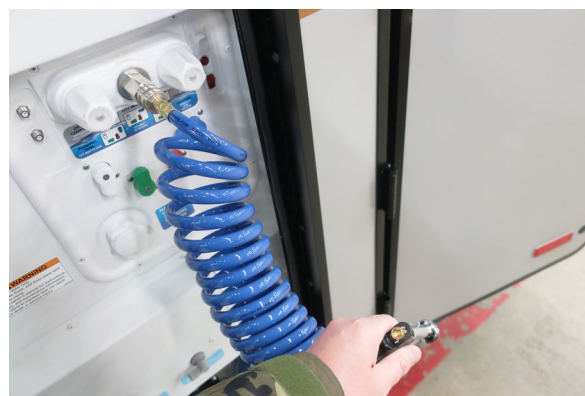
Exterior Shower/Wash Station (located in the drivers side service center, shown with shower hose hooked up. -Typical View)
