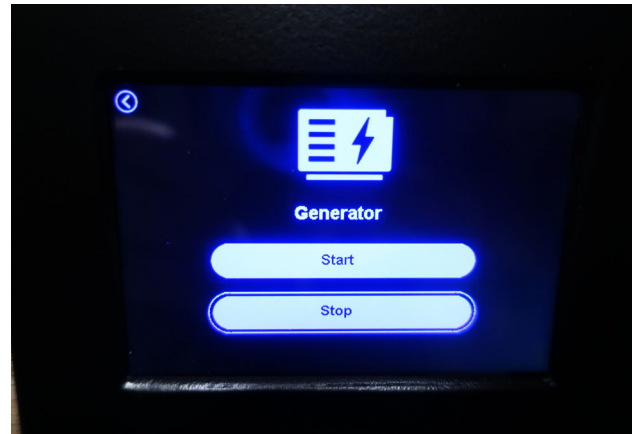
Select the Generator Icon on the main menu to access the Generator start/stop screen. -Typical View
