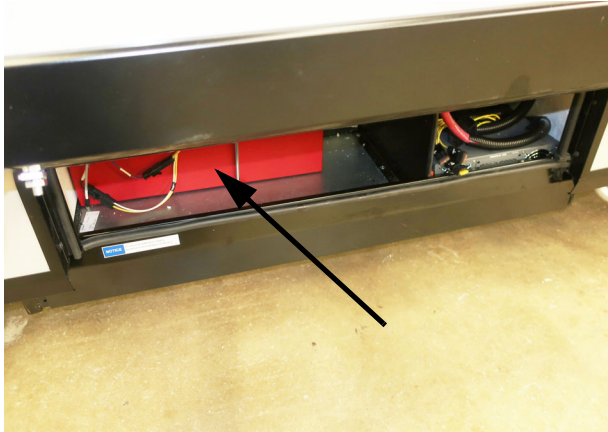
Battery (Located inside drivers side exterior door) -Typical View
