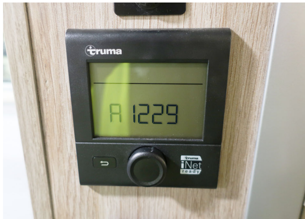
Water heater controls located next to the bathroom door. -Typical View
