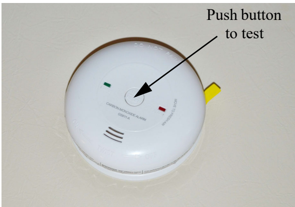
Carbon Monoxide Alarm
