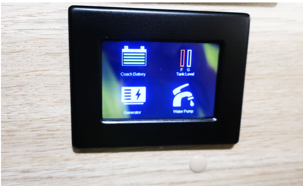
System Monitor Panel -Typical View
