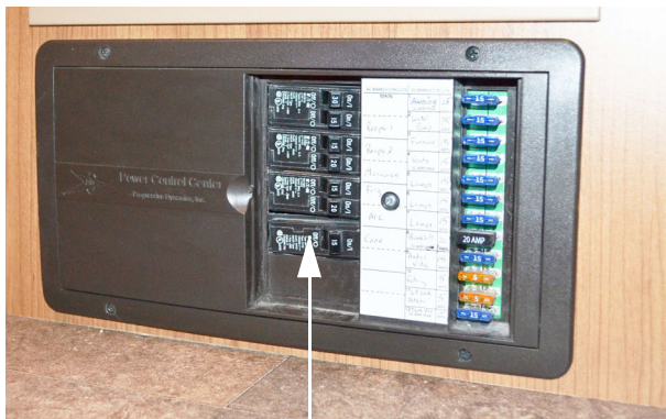
120-Volt Circuit Breakers -Typical View
