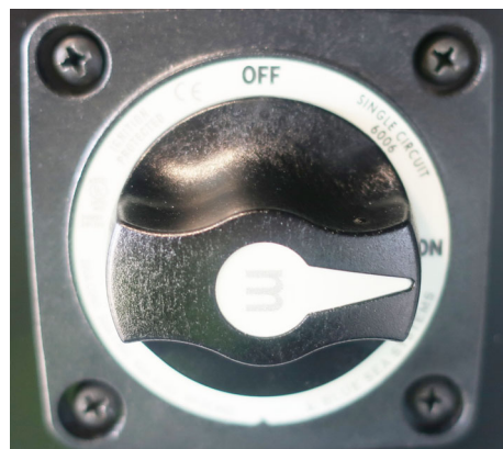
Inverter/charger disconnect switch. (Located inside the passengers compartment door near the Charger Unit) -Typical View
