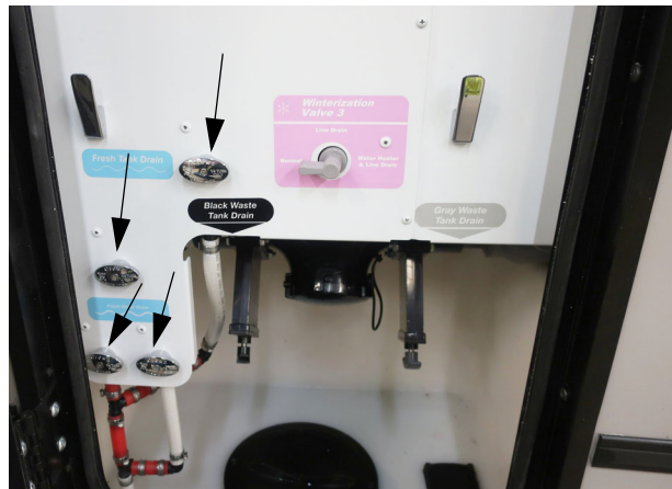
Waterline drain valves (Shown in the closed position turn valves to open). -Typical View
