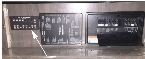
House Circuit Breakers -Typical View
