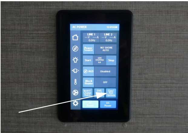
Generator Switch and Hourmeter (Located on multiplex monitor panel “AC” Screen) -Typical View
